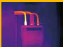
Poor connection and internal damage
