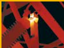
Incorrectly secured connection
