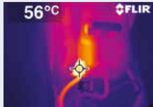
What a thermal imaging camera sees.
