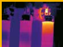
Internal fuse damage
